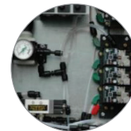
Pneumatic control systems
